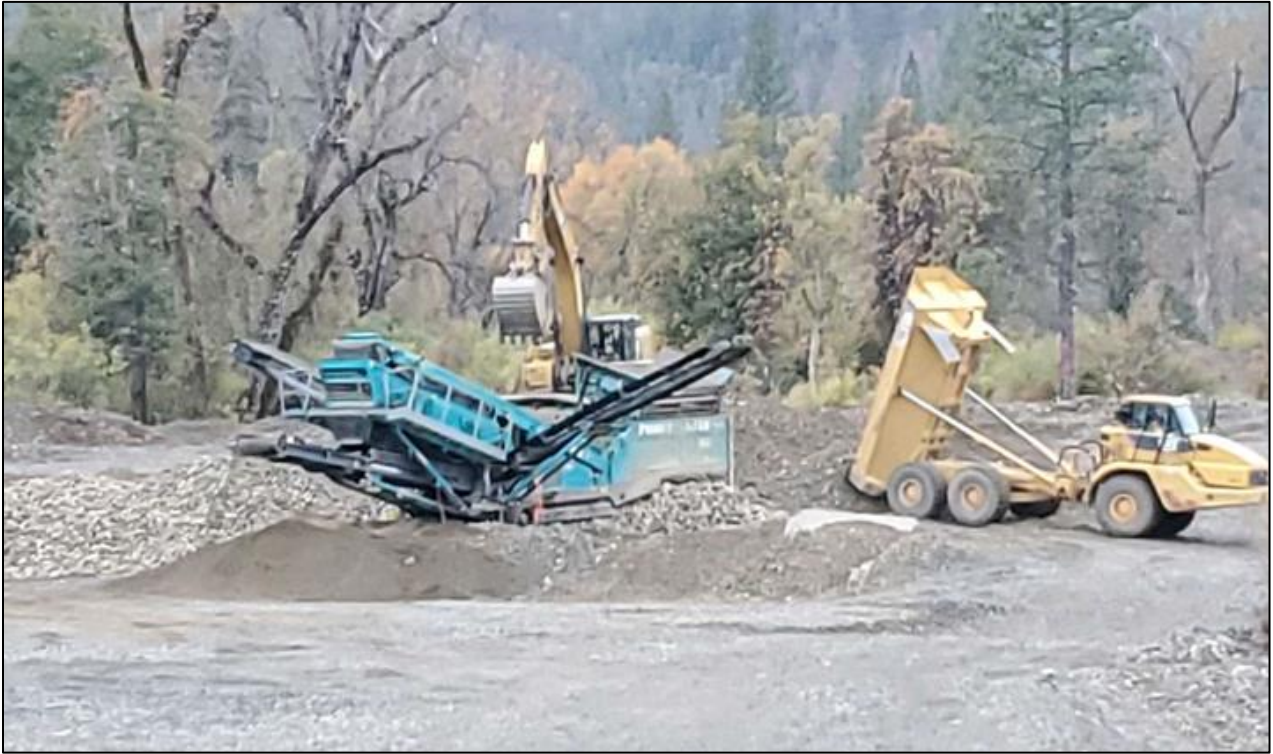
Figure A-3. Sediment processing equipment at a restoration site, including a belt conveyor, front loader, excavator, and screening plant to sort materials by size class.
