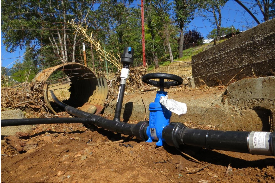
Figure 7: Gate Valve with HDPE fusible ends and Netafim 1" Combination Air/Vacuum and Continuous Acting Air Vent installed at existing overflow structure. Vents allow for discharge and intake of large volumes of air along mains and at the end of mainlines and provide continuous air release at high points in pipe network or upstream of manifolds.
