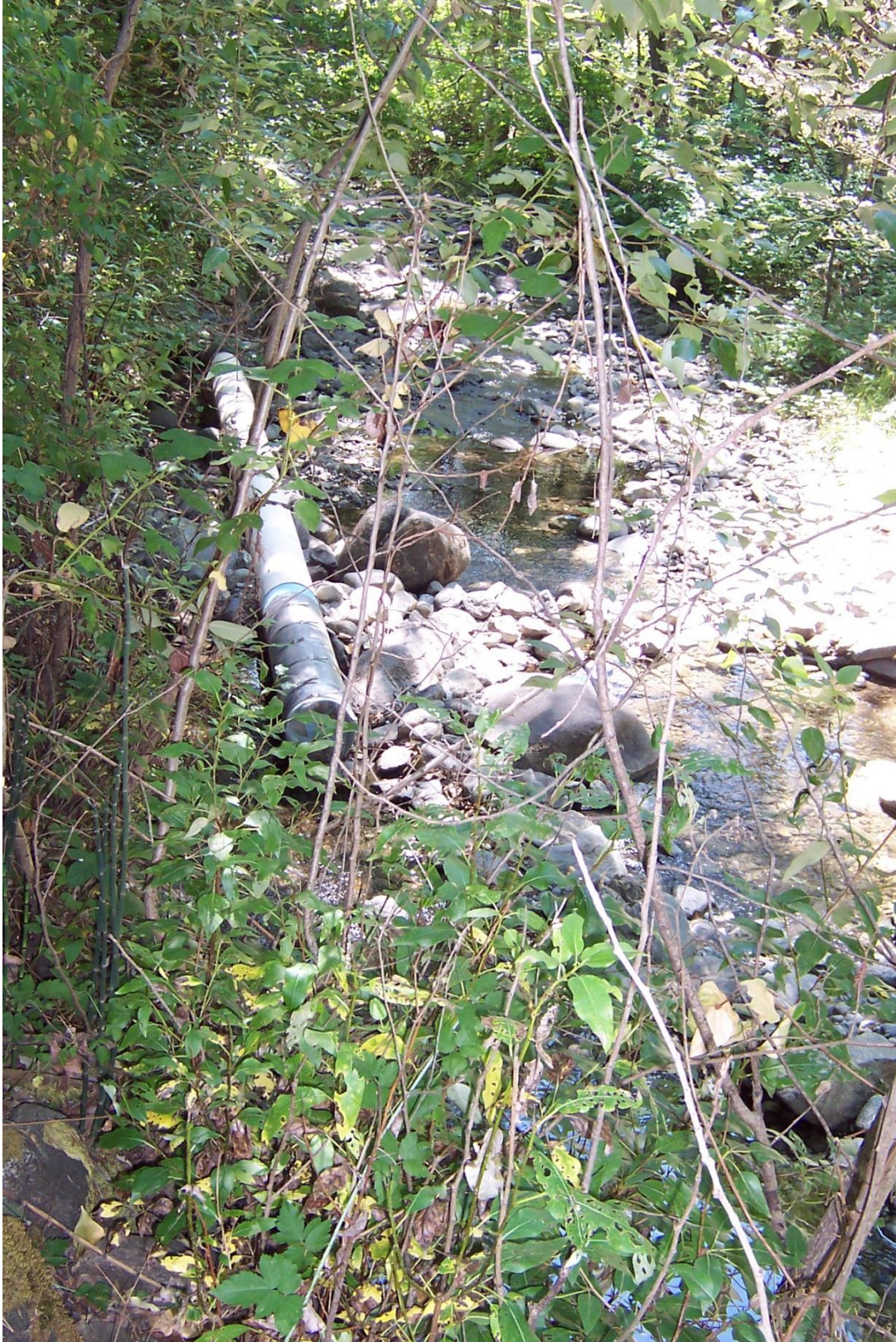
Figure 4: Existing East Weaver Creek Intake Structure had deteriorating pipe and materials.
