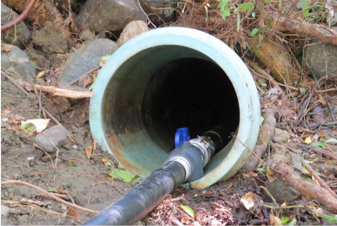
Figure 61: New HDPE Butt-fusion intake pipe with quick-disconnect cam-lock fitting and shutoff valve utilizes portions of the existing East Weaver Creek Intake Structure thus minimizing disturbance to the streambed and bank.
