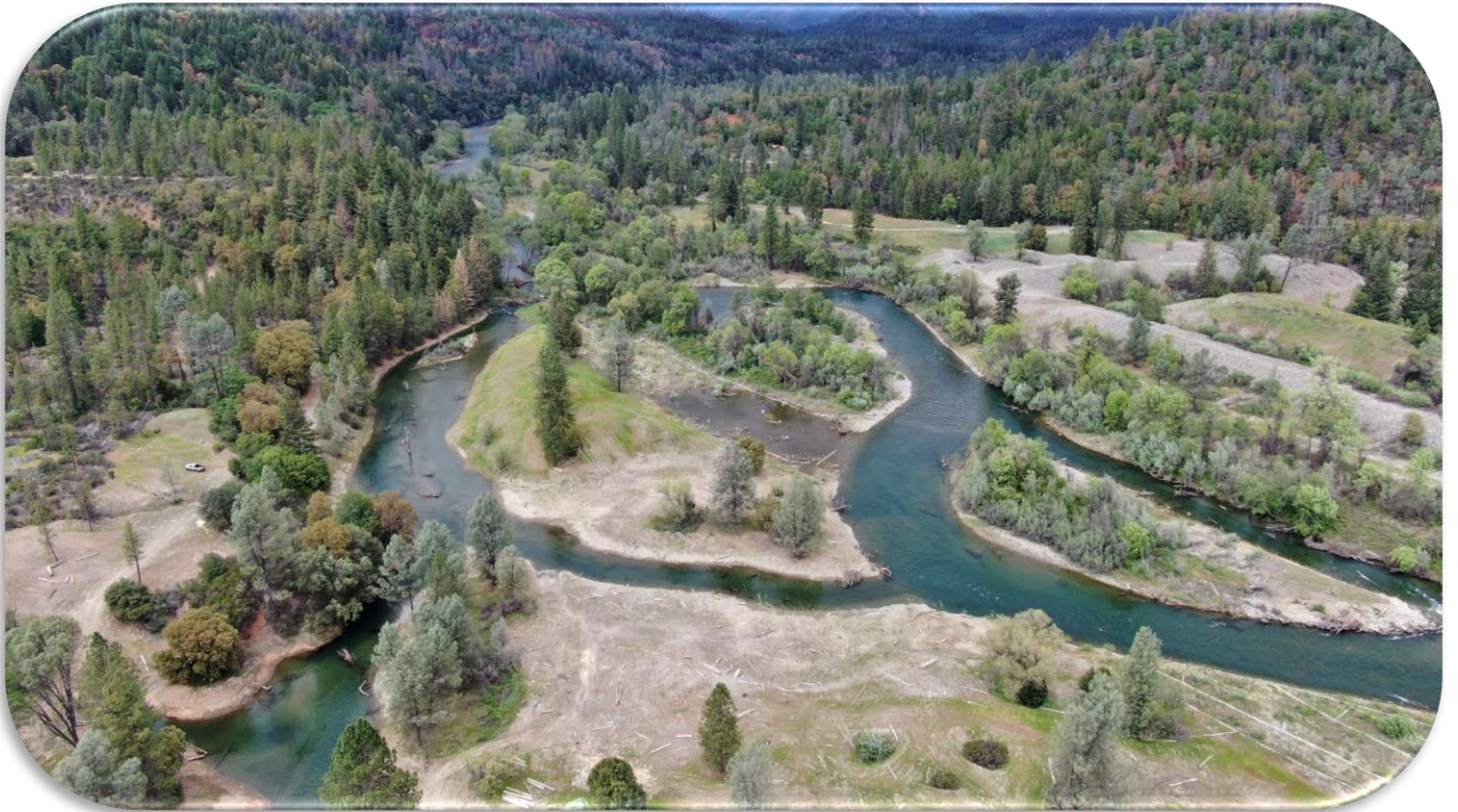
Aerial view of Chapman Ranch site after construction (Aaron Martin, Yurok Tribal Fisheries Department)
