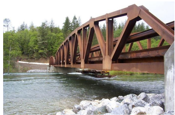
Salt Flat bridge after infrastructure improvement with a flow of 6000 cfs. The old bridge can be seen in the background to the right. (TRRP)
