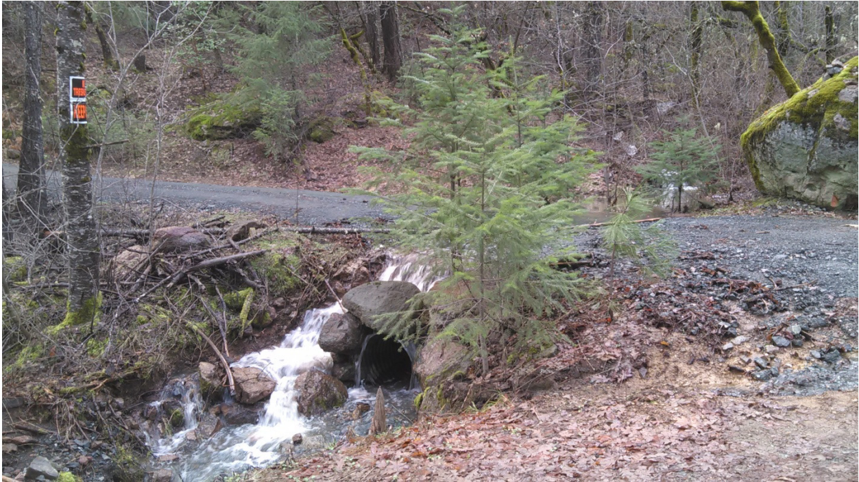
A stream overtops the culvert but does not divert out of the crossing.
