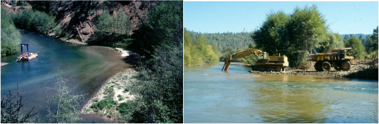
Figure 27: Suction dredging in Stott Hole in 1977 (left). The area occupied by the sand bars on the right side of the photograph is currently about 20 ft deep. Right: Pool dredging with an excavator.
