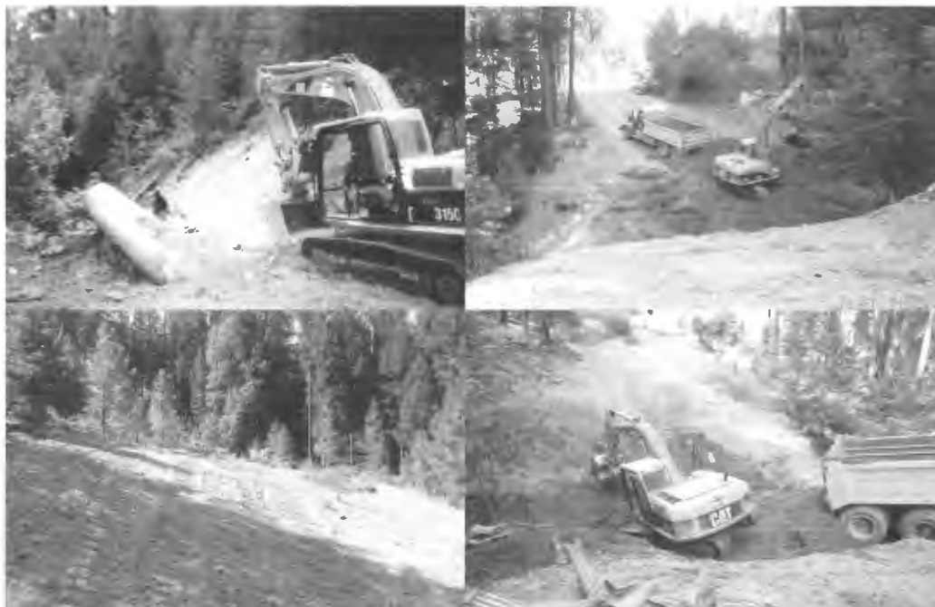
Figure C. This set of 4 photos shows typical decommission activities including; removing a CMP and fill at a stream crossing and ripping/outsloping a road.
