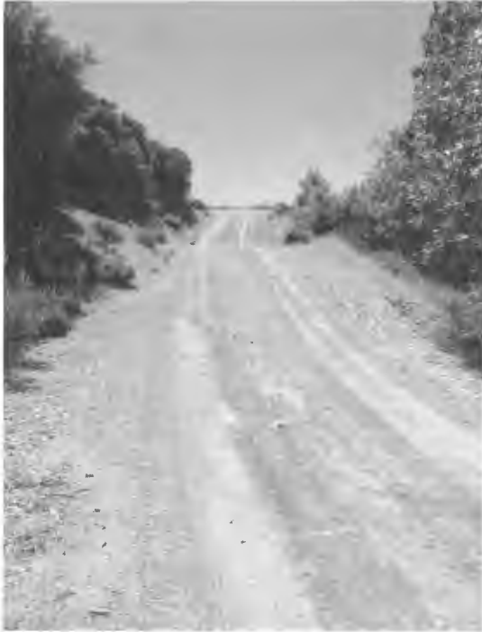
Figure N. Photo of rolling dip on road 31N38.
