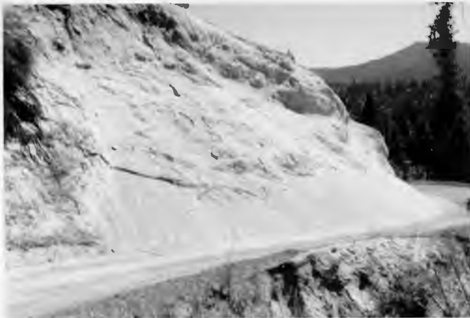
ROADBANK IN DECOMPOSED GRANITE BUCKHORN DAMSITE WATERSHED
