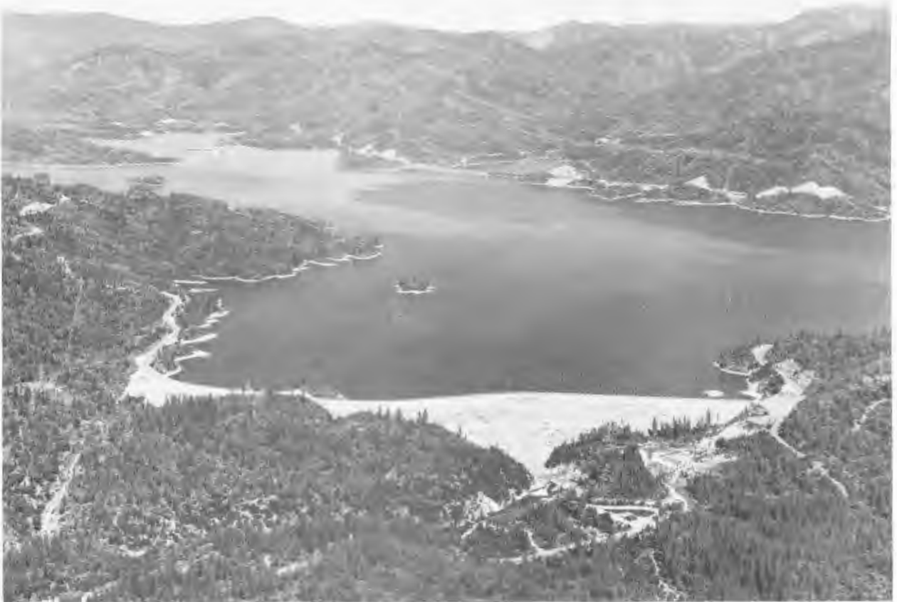
Aerial view upstream of Whiskeytown Dam and Lake. Note vehicular road traversing the earthfill dam across the lower central area of the photograph.
